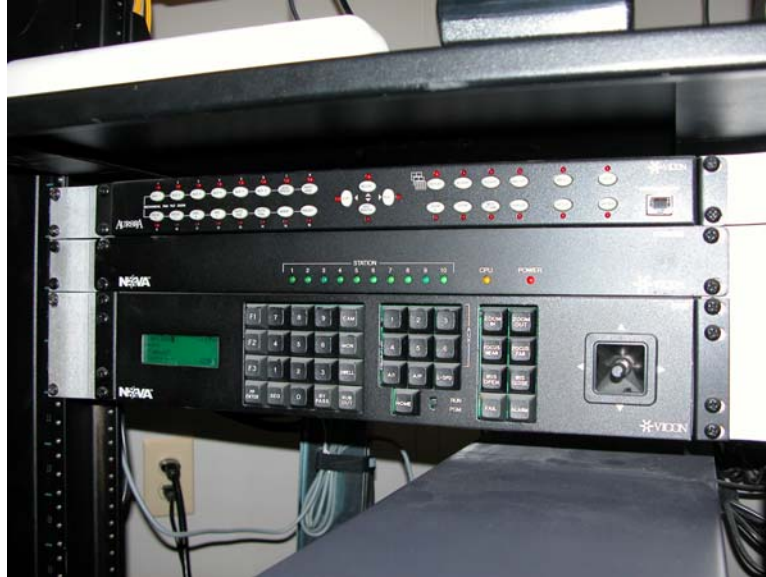
Figure 4.5 – CCTV Control CPU and Multiplexer Panel
