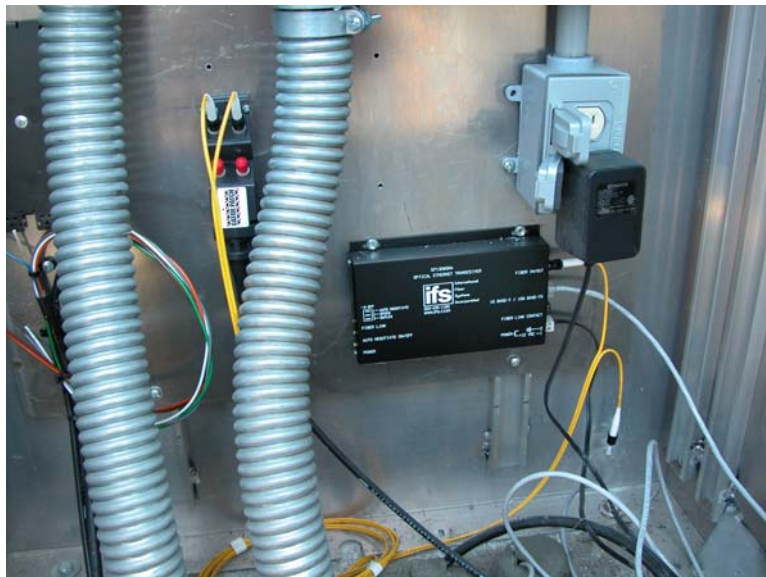
Figure 4.9 – DMS Site Field Cabinet Fiber Transceiver
