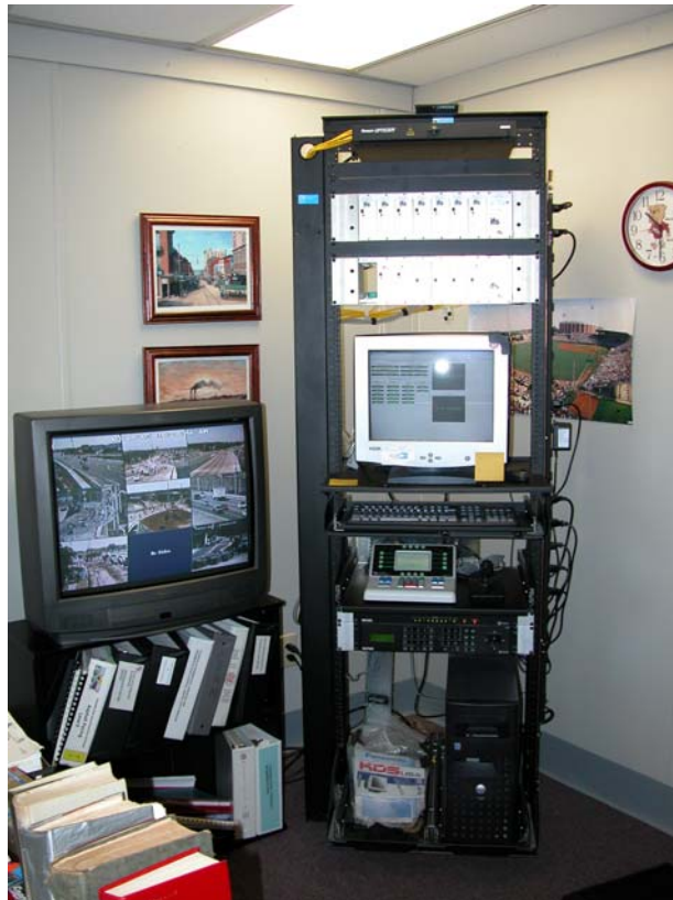
Figure 4.4 – Metric Engineering Field Office Command and Control Room
