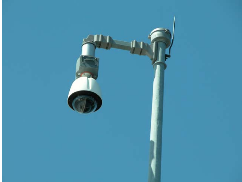
Figure 4.12 – Hathaway Bridge Camera and Lowering Device
