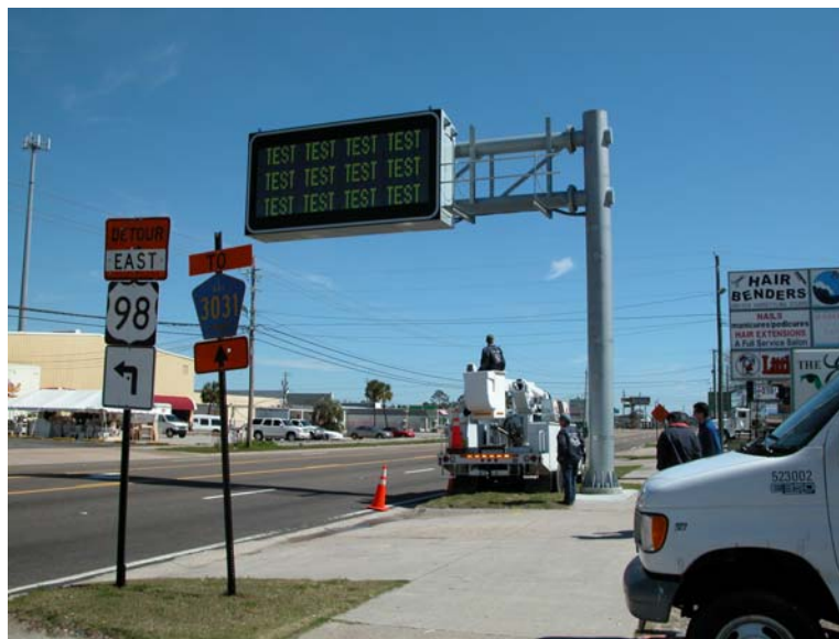
Figure 4.7 – DMS Installation Location
