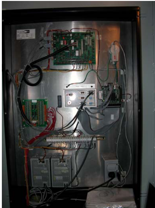
Figure 4.10 – DMS Controller and Panel inside the Sign Cabinet
