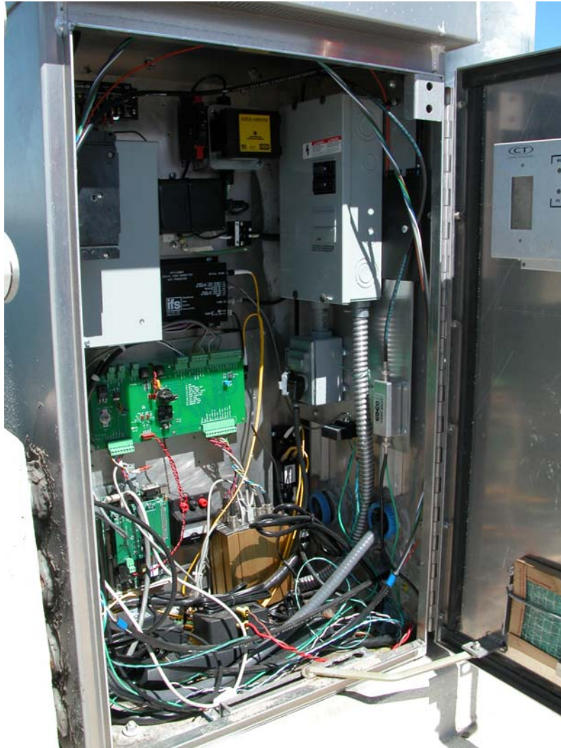
Figure 4.14 – RWIS / CCTV Cabinet VIEW 1
