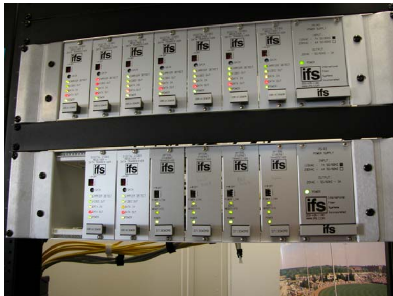
Figure 4.6 – Fiber Optic Transceivers
